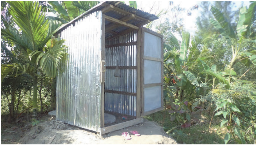
Fig. 6.8. Single pit latrine, where the super-structure is built by the stakeholder and the sub-structure by DPHE, Noler Char.
