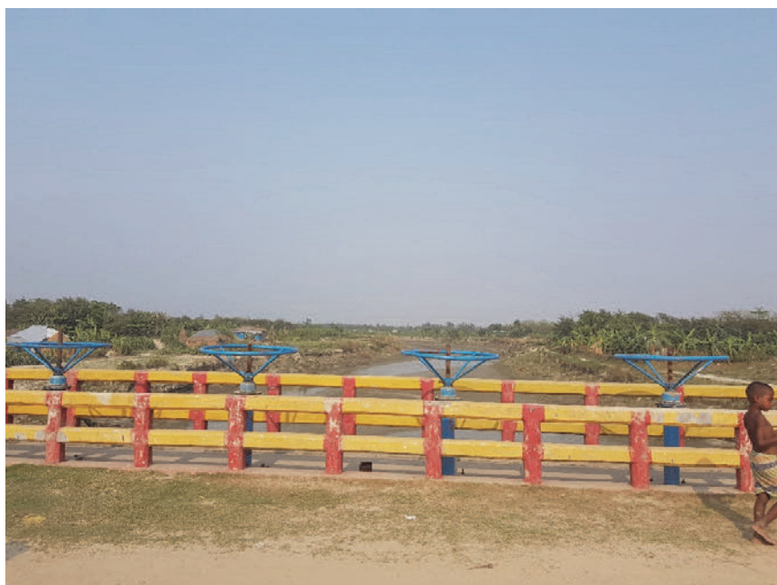
Fig. 6.3. Lift gate operating deck at C/S of Sluice DS-1, Char Nangulia.
